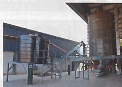
The installation allows grain from the intake pit to by-pass the dryer and be sent straight to the store on rare occasions when moisture content is low enough.
