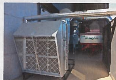
Air is pre-heated to 85°C by passing through a heat exchanger before entering the dryer, saving time and fuel.
